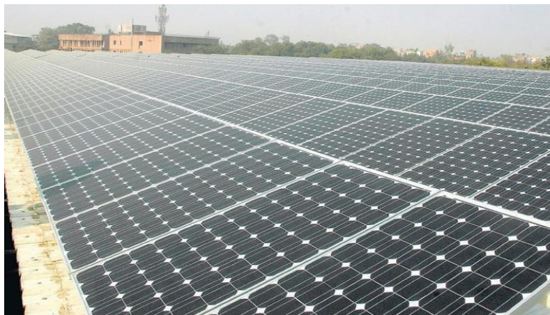
Fig: 7 Solar Plant of Neemuch, Madhya Pradesh
